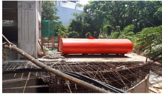
Figure 1: A typical tank
